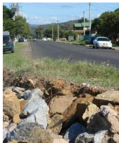
Wharf Rd where rock was dumped to try to prevent the road being washed away. Part of the development site is on the right (with construction fencing)
