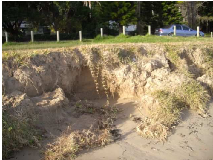
Recent erosion at Long Beach caused by large waves and high tides
