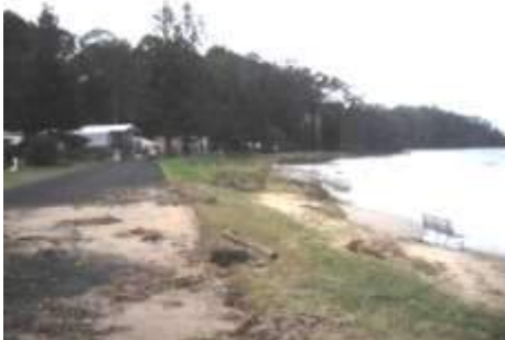
June erosion at Long Beach removed some of the reserve and damaged the road.
